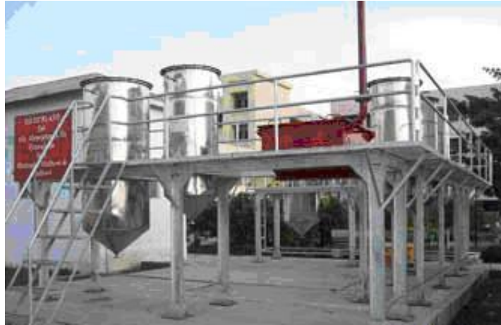
A working plant to Capture CO2
